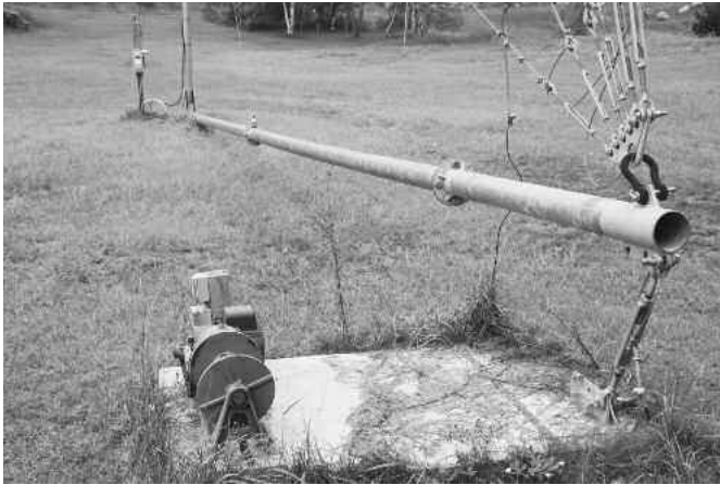
Fig. 6.12: Gin Pole. The gin pole is attached to the anchor. Notice the electric winch to the left of the attachment.
