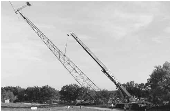
Fig. 6.5: Crane Lifting Tower and Turbine. This 80-ton crane lifts a massive turbine and tower into place. The hinges at the base of the tower allow the crane to tilt the tower into position.
