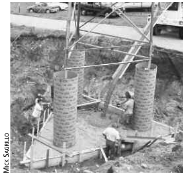
Fig. 6.4: Concrete Piers and Base of Tower. This massive, deep foundation supports a 120-foot freestanding lattice tower. Each leg of the tower will attach to a steel leg embedded in each of the vertical piers. The piers and base of the foundation are made of concrete reinforced with rebar.
